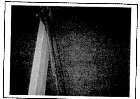
Sample No. 50725CB013 Location R001 Description Roof felt
